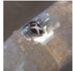
The wire mesh reinforces the repair area and forms a mechanical backing for the epoxy.
